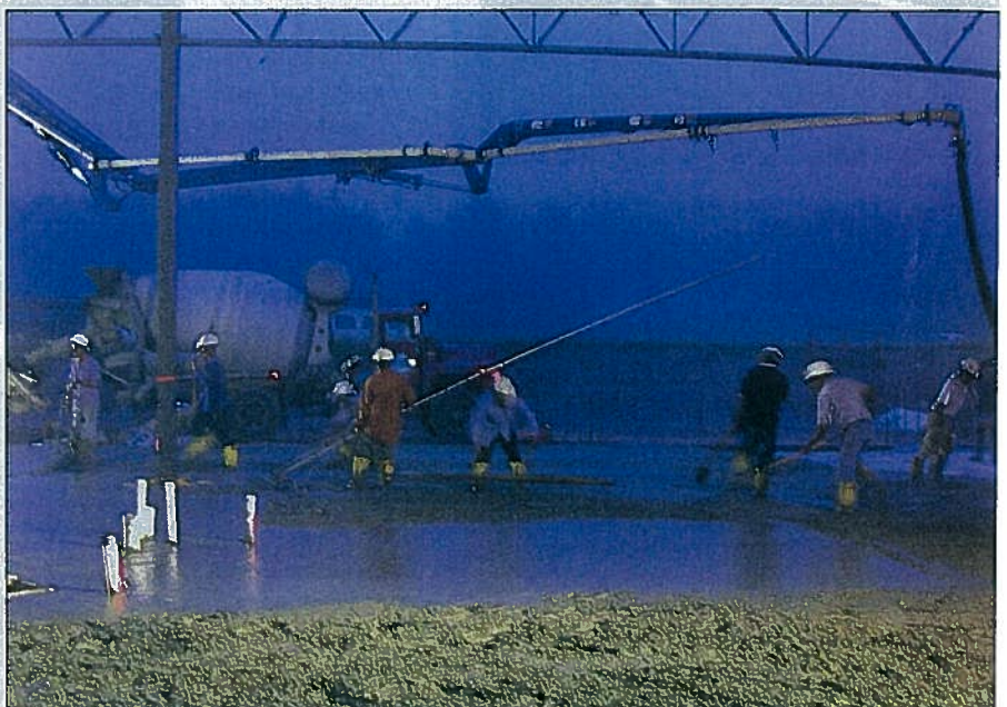
Bartley Contracting gets to work early in the morning pumping a slab that includes a new synthetic structural fiber.
