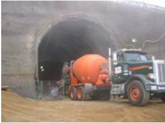
FORTA-FERRO ® -reinforced tunnel lining for Clo de la Tech Winery in California
